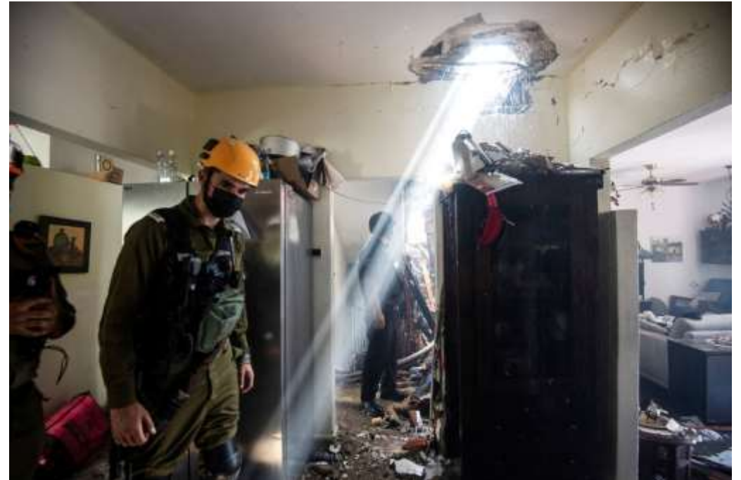
Building in Ashdod, southern Israel, damaged by a rocket launched from the Gaza Strip on May 11, 2021. Avi Roccah / Reuters
