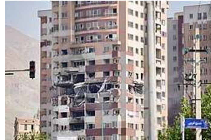
A residential building in Tehran with missile damage, 13 June 2025
